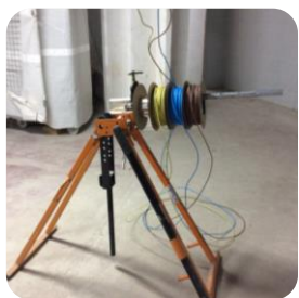
Inadequate Cable Rollers
