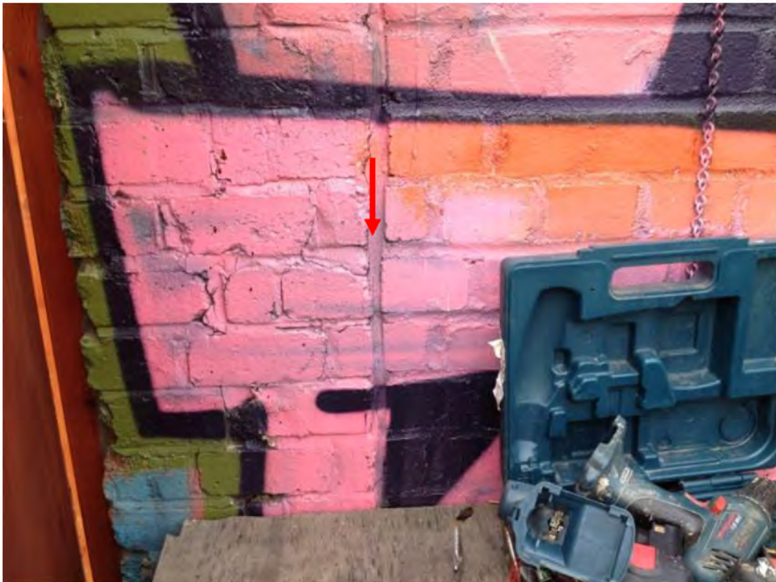
East end of boundary line – outer wall. The joint between the buildings is exactly 25.65m from the South East building corner
