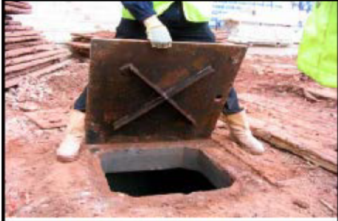
Temporary access chamber cover in trafficked area Note fixing hole in plate & cruciform to allow positive location in opening
