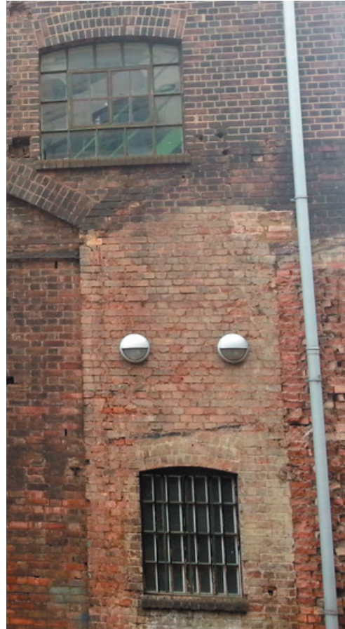
Part of the west elevation showing the existing metal windows and the residual marks left by previously demolished buildings
