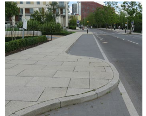
Pre-cast concrete (PCC) raised kerb and flush kerb at carriageway edge - North Park edge
